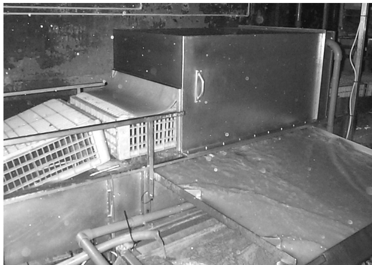
Figure 5: Pre wash booth and associated water recirculation equipment. The run down screen that filters the water is just out of view from the bottom right of the photograph. Screened water collects in the main tank from where it is recycled to the jets in the booth and to the soak tank. Make up water is added to this tank.
