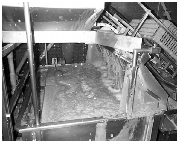
Figure 9: Crates leaving the soak tank to enter the main wash module (bottom corner only visible in top left of photograph). Water carried over by the crates and the drainage water from the wash booth falls back into the main water tank via a run down screen. The ball cock controlling the make up water is visible in the centre of the photograph.
